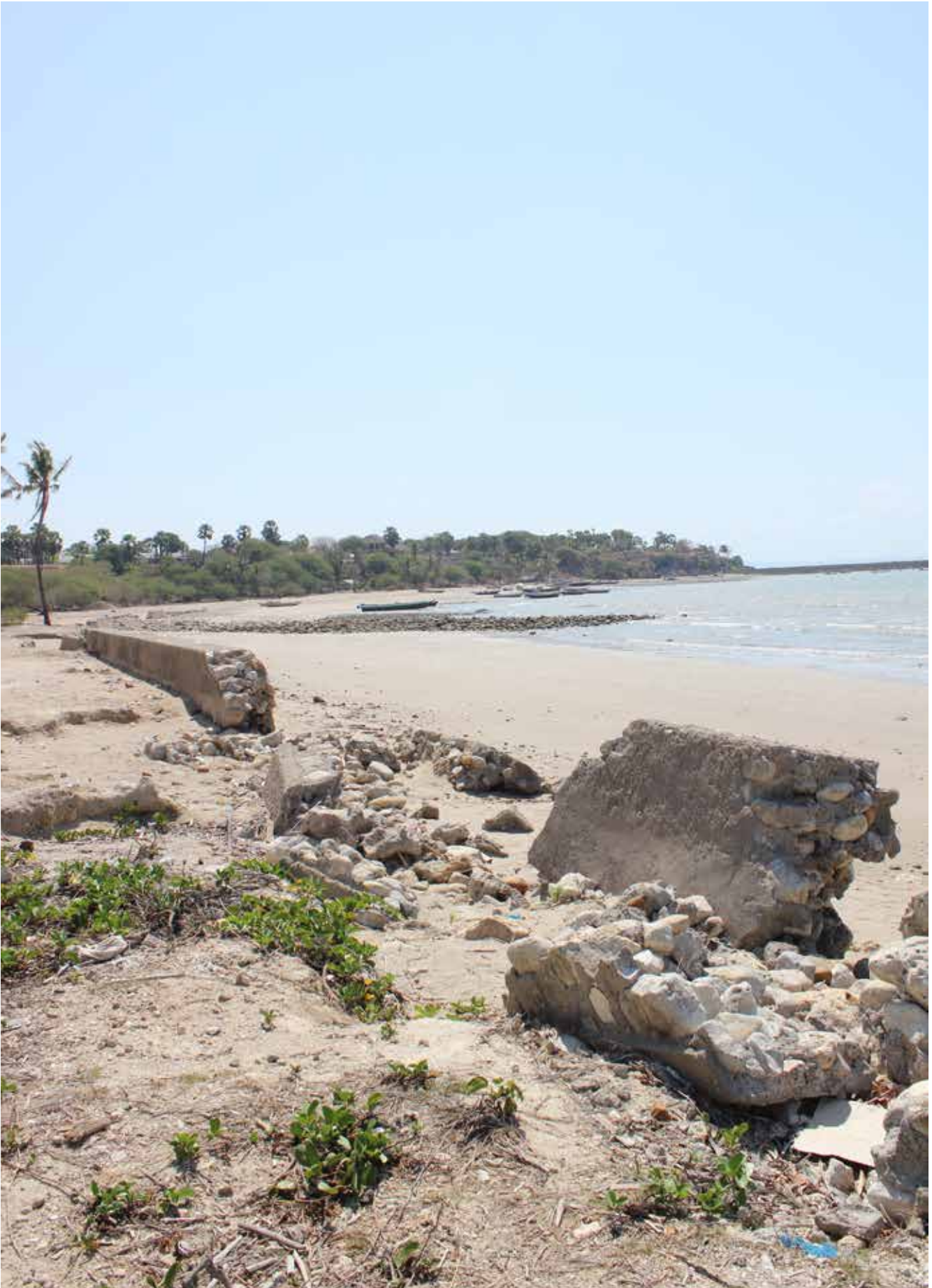
Figure 24. The impact of abrasion of coastal areas is already present. Damaged sea-walls demonstrate how they have limited success in blocking the destructive power of the sea, so other solutions are necessary. Replanting mangroves is a possible solution that can be implemented with the help of coastal communities themselves.
