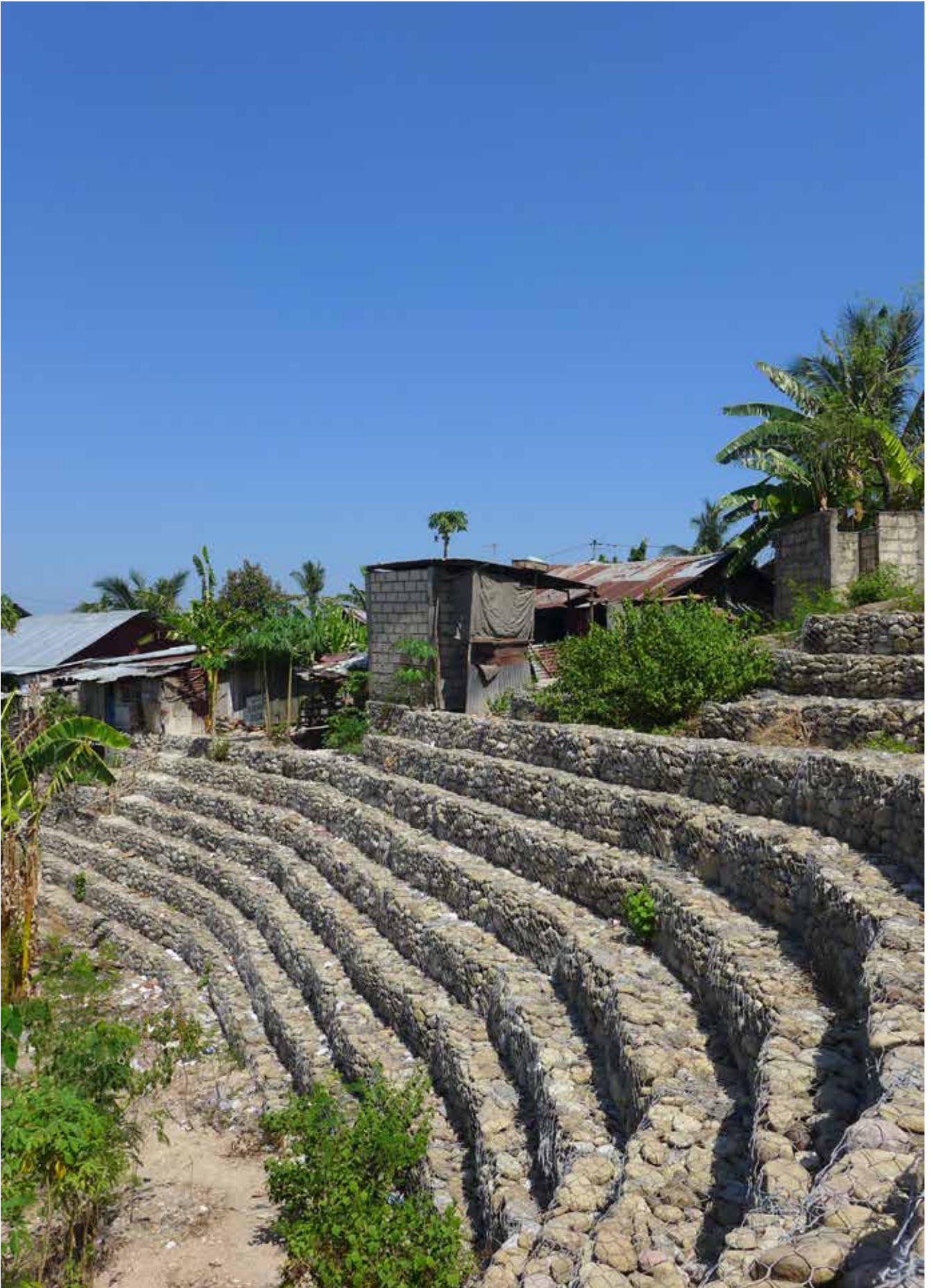
Figure 21. An example of a good practice to reduce vulnerability in areas which are prone to landslides. The construction of retaining walls made of gabions prevents landslides, and protects people, their homes, and property during the rainy season.
